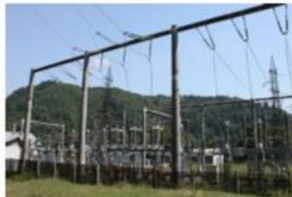
Power generation and distribution
